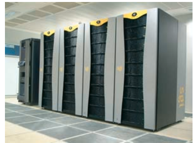
COSMOS (Mark VI), the UK National Cosmology Supercomputer housed in DAMTP.
